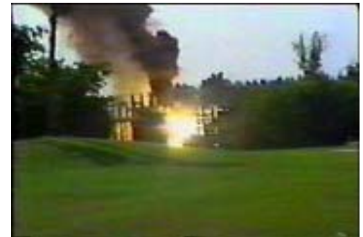
Uncleared short circuit in substation. (Click photo for 5MB mpg QuickTime footage, about 30 secs.)
